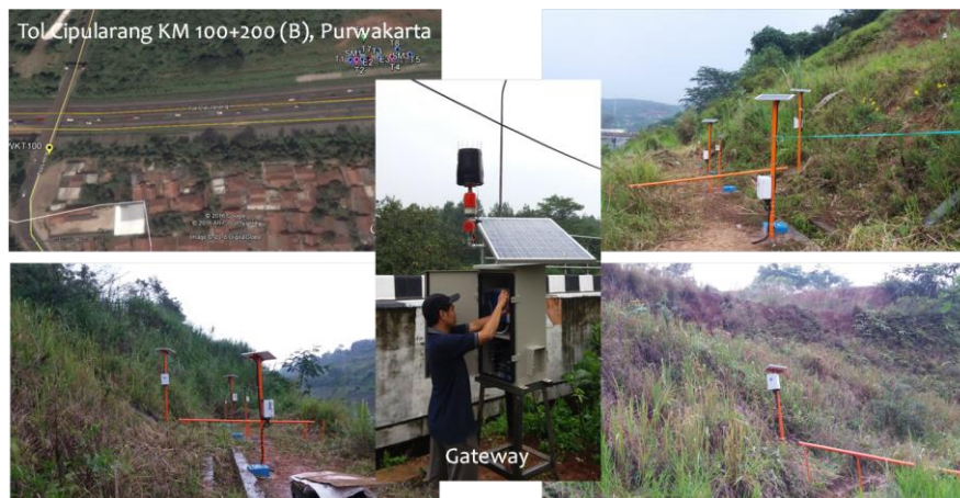
Fig. 2. Prototype of WISE-LAND installed at Cipularang toll road KM 100, Purwakarta District, West Java. The system consists of 4 sensor modules, 4 wire extensometers, 8 tiltmeters and 1 gateway with raingage and alarm.
